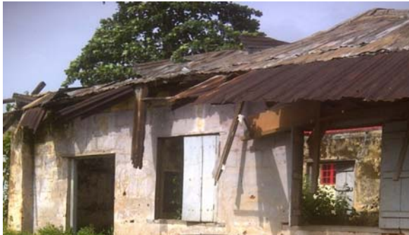
Fig. 3: The existing schools in the community are in a state of disrepair
