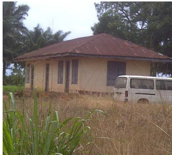
Fig. 4: The primary health centre in the community appears unused as it is overgrown with weeds
